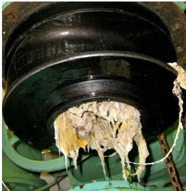
Pipe Clogged by Wipes
