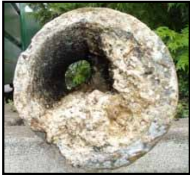
Grease clog in a sewer pipe
