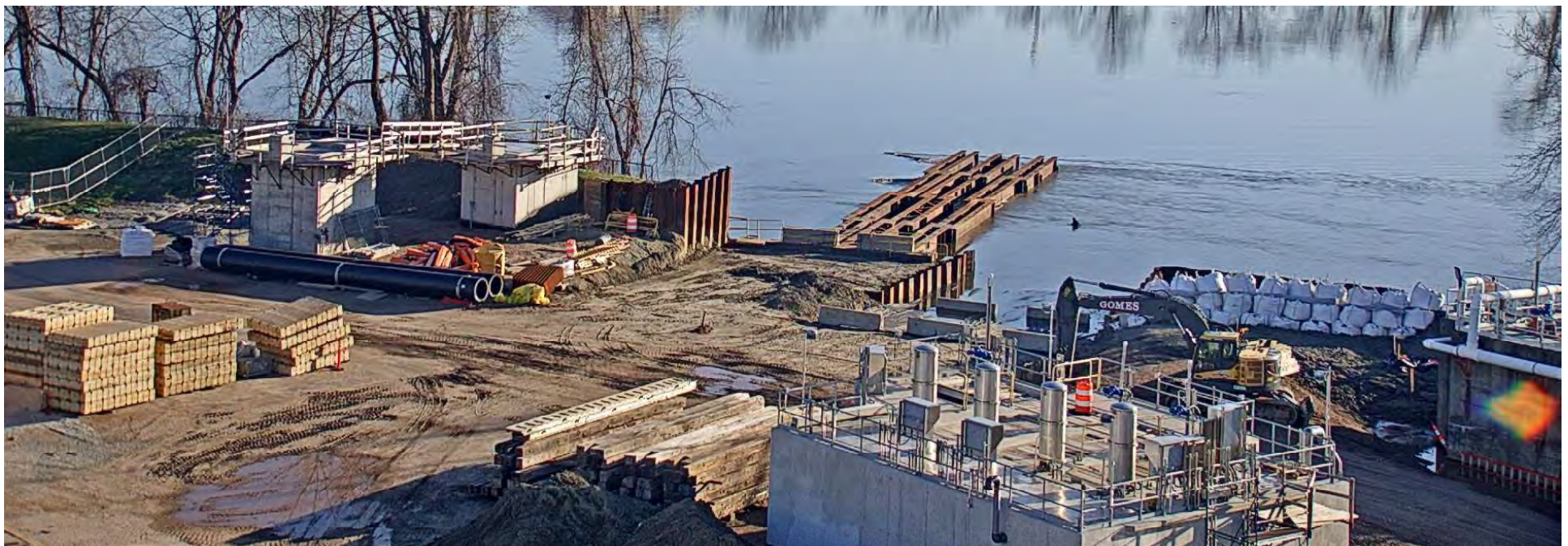
Top: Crews work on the preliminary stages of the York Street Pump Station dock on the Connecticut River in June 2021; bottom: the dock is being built in October 2021.
