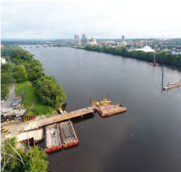
Top: The Commission conducts high-pressure cleaning in sewer pipes. Bottom: Construction of the temporary pier to support construction of the new river crossing project is well underway. The City of Springfield is pictured in the distance.
