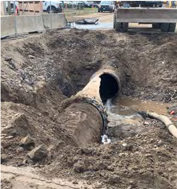
Top and Bottom: Crews responded to a water main break on East Columbus Avenue in August 2020. The broken main dated from 1909.
