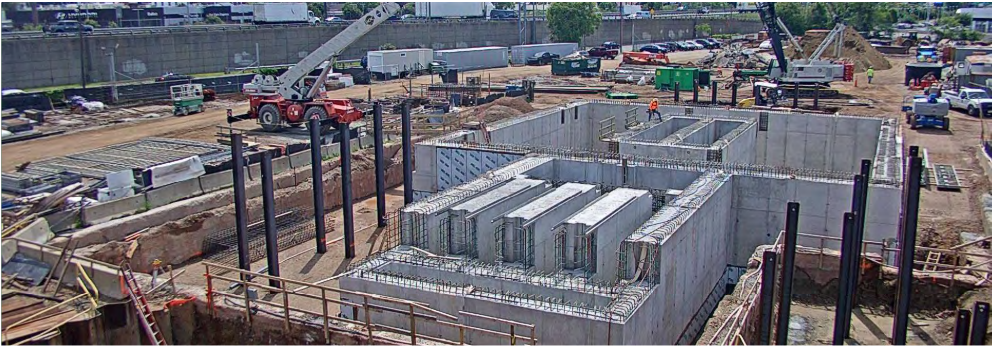
The York Street Pump Station's foundation is poured in November 2020, top , and June 2021, bottom .
