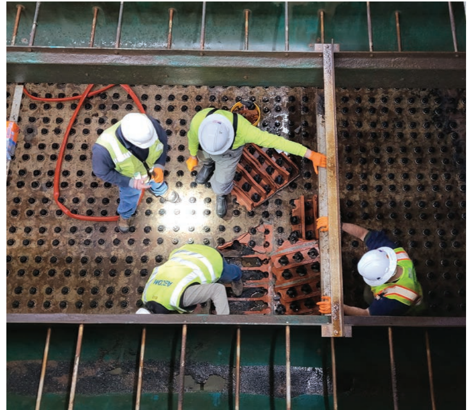
Rapid sand filter #6 failed during a routine backwash in January 2021.
