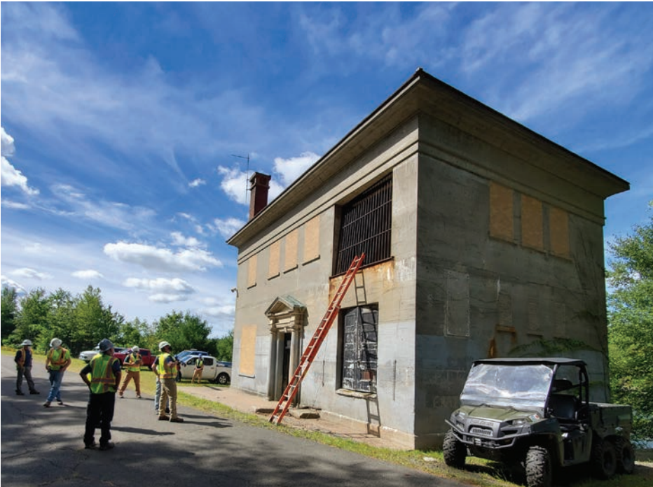
The Diversion Gate House receives upgrades to expand its use to year-round.
