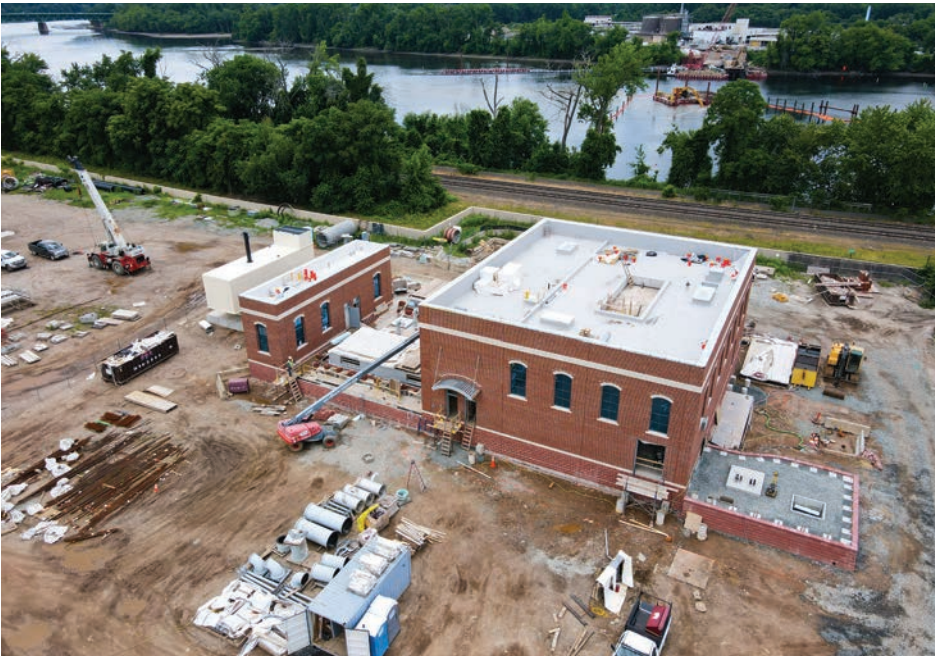
Top: Progress is made on the York Street Pump Station in June 2022. Bottom and top right: Aerial views of the York Street Pump Station and Connecticut River Crossing Project in August 2021.
