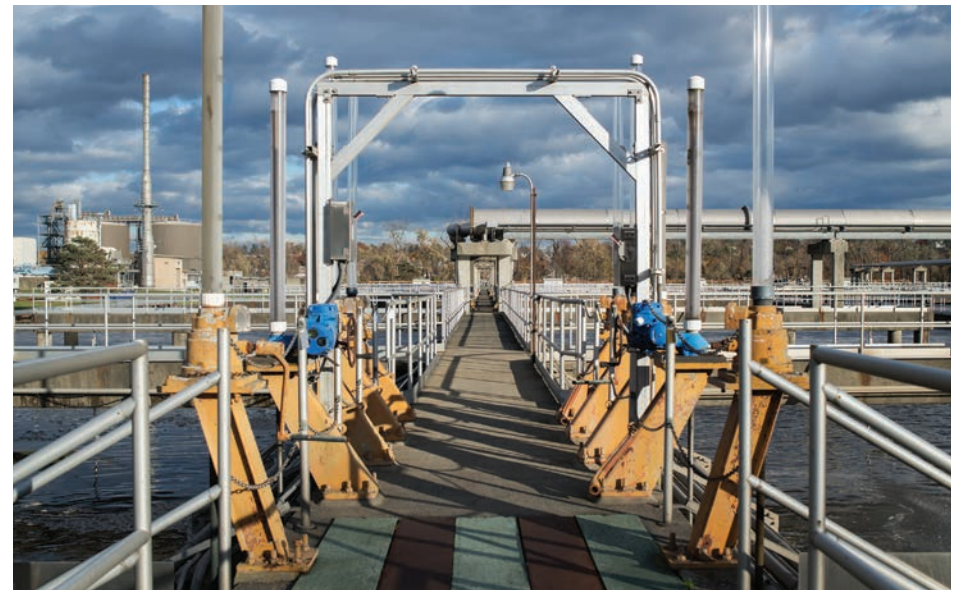
Top and bottom: Views of the aeration basin (secondary treatment) of the wastewater treatment plant.
