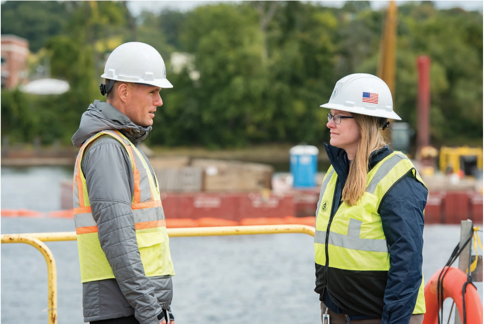
Director of Engineering Darleen Buttrick (right) confers with a colleague at the site of the Connecticut River Crossing Project.
