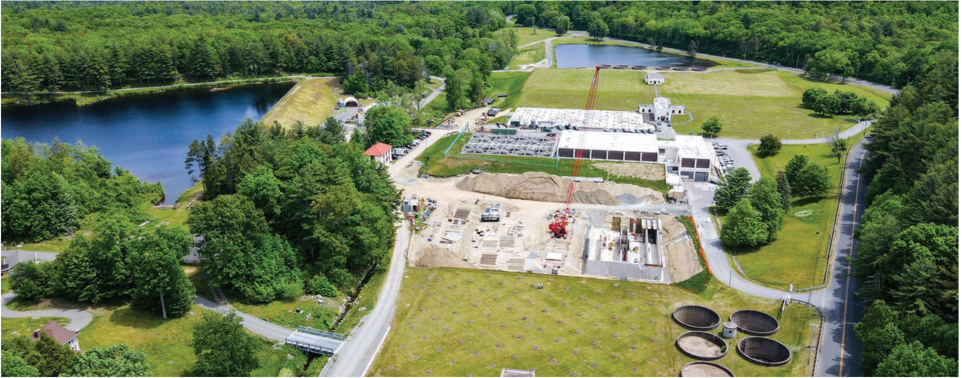
An aerial look at West Parish Filters Treatment Plant, with the new Clearwell and Backwash Pump Station project (Phase 1 of the new plant) under construction in summer 2021.
