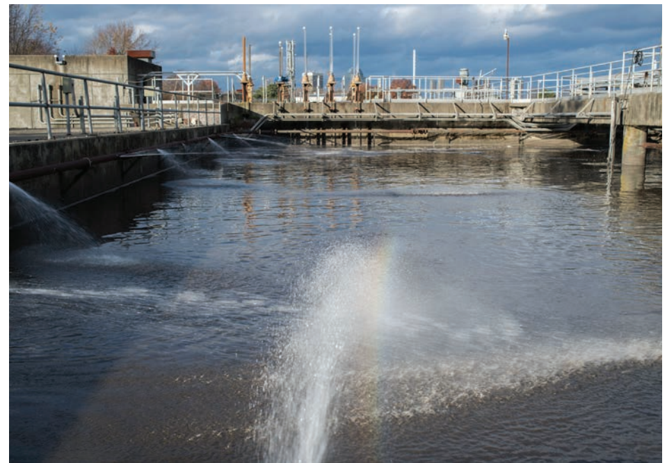
Top and bottom: Scenes from the Springfield Regional Wastewater Treatment Facility on Bondi's Island.
