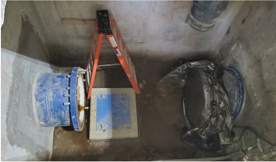
The 42-inch-diameter valve is being replaced to help ensure redundancy for water flow from the reservoir to the West Parish Filters Water Treatment Plant.
