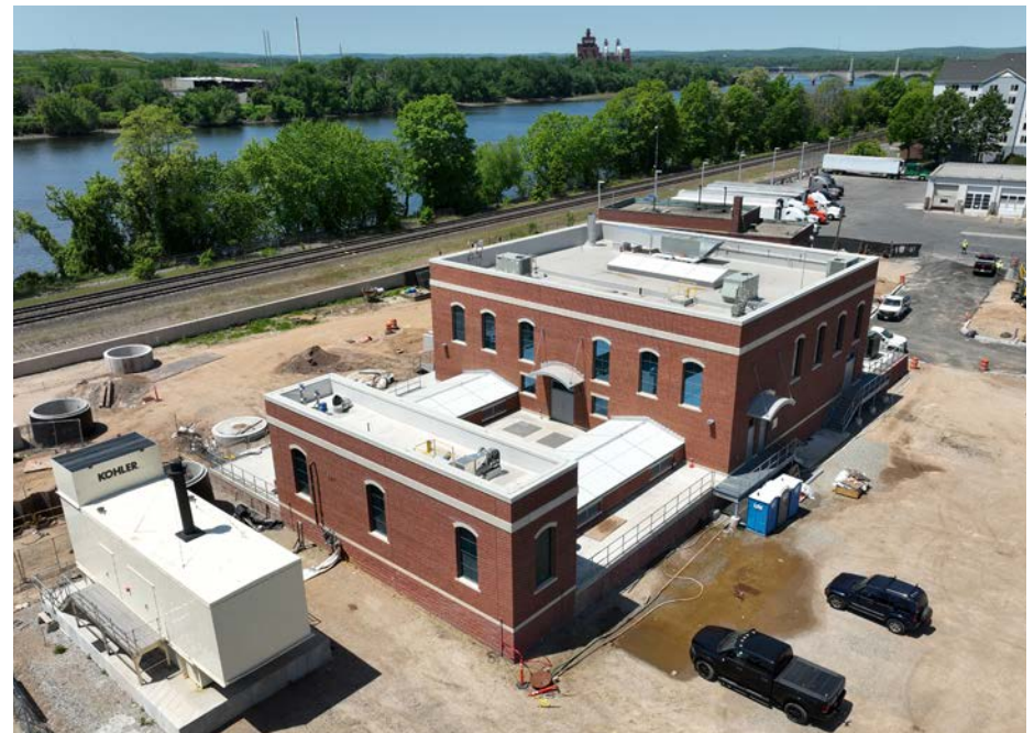
Left and top: Views of the SRWTF, including the secondary treatment aeration basins undergoing rehabilitation (left), and the restored riverbank (top) from the river crossing work. Bottom: The new York Street Pump Station nearing completion.
