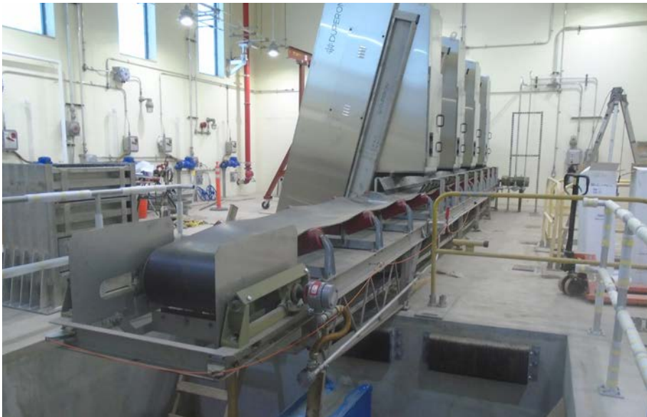
Top to bottom: The new York Street Pump Station pumps and screening room.
