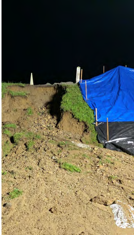
Dam #2 Slope Partial Failure, 2021
