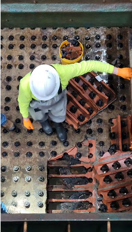
Rapid Sand Filter Drain Failure, 2021
