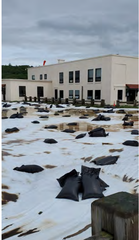
Temporary Clearwell Tarp, 2021
