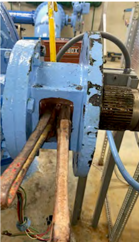
Backwash Actuator Valve Failure, 2020
