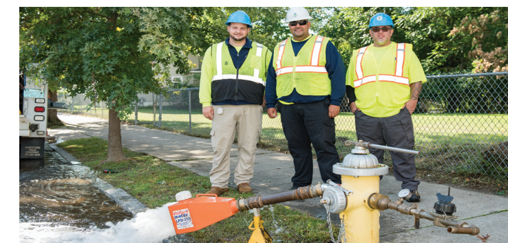
Field Service crews maintain more than 500 miles of pipe and over 6,000 hydrants within the distribution system in Springfield and Ludlow.
