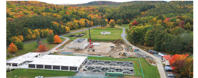
Phase 1 Construction: The new clearwell under construction at West Parish Filters Water Treatment Plant in October 2022.
