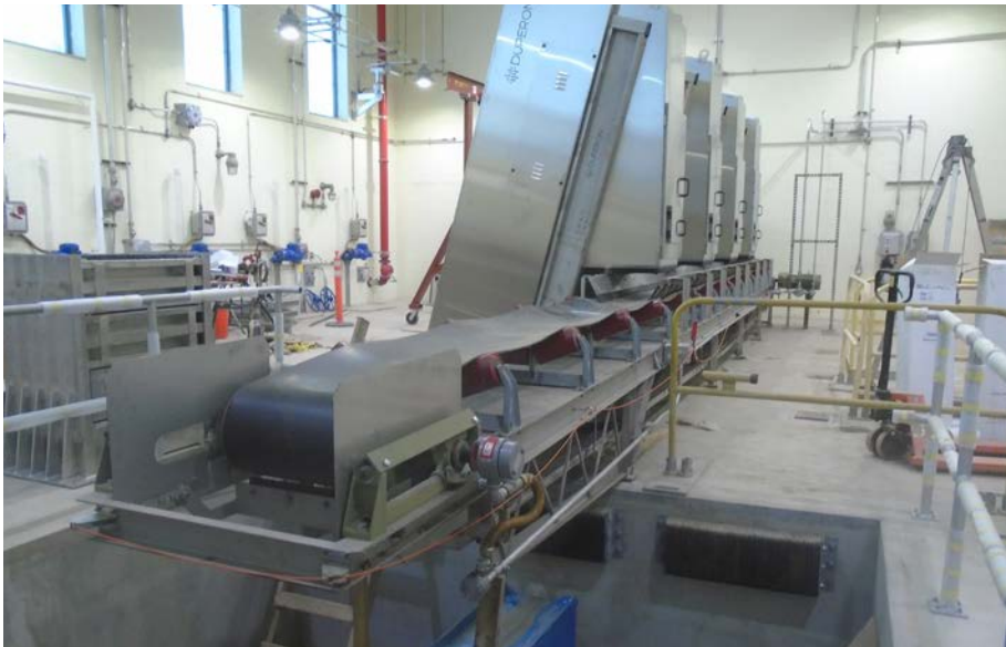
Top to bottom: The new York Street Pump Station pumps and screening room.
