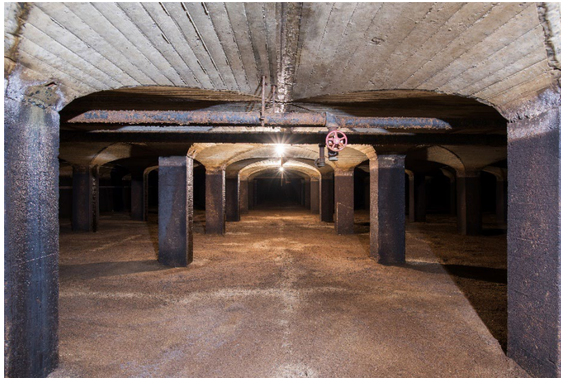
Slow sand filters, built c. 1925, are still in use at West Parish Filters Water Treatment Plant
