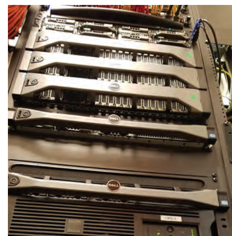
Below: Upgraded server equipment was installed to better handle data storage and transmission across the Commission network.
