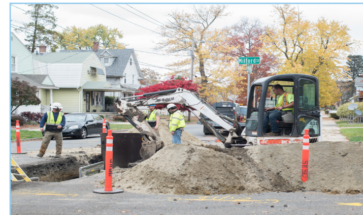
Commission crews replace a water main on Milford Street in Springfield (above). WIFIA financing will support additional water main improvement projects within the distribution system.
