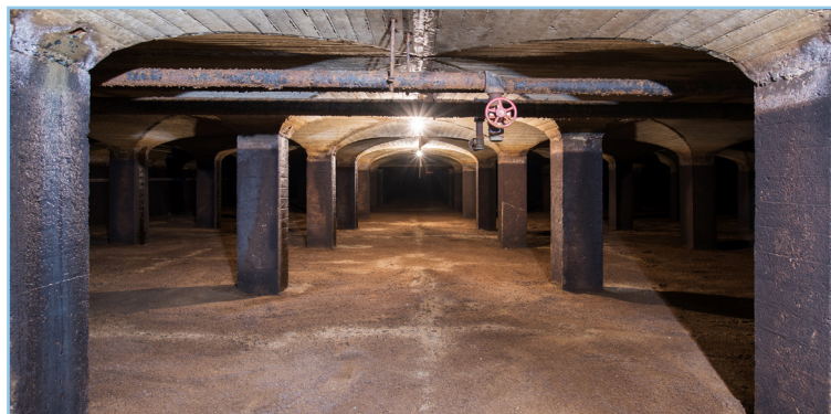
Pictured above is a 1920s-era slow sand filter, still in use today to meet peak demand. All slow sand filters will be eliminated upon construction of the new treatment plant.
