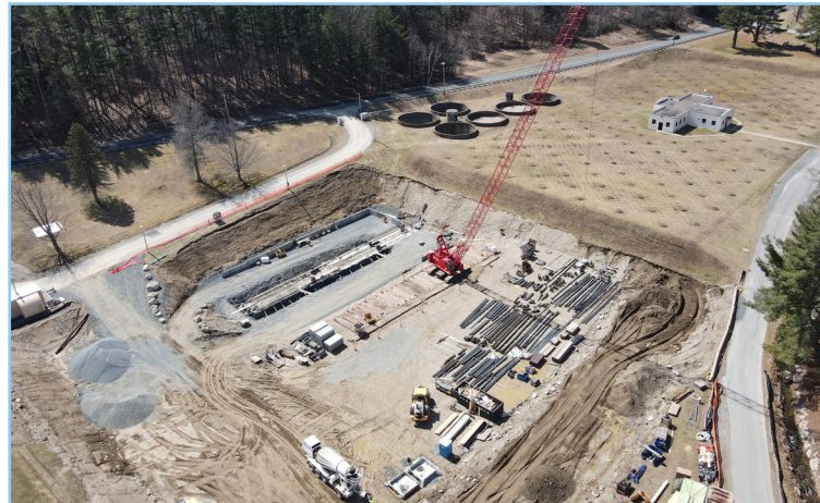
In 2021 the Commission broke ground on a new era of drinking water treatment at West Parish Filters. Phase 1 construction of the new water treatment plant is currently underway, with construction of the new Clearwell and Backwash Pump Station Replacement Project. Original 1909 slow sand filters were demolished to make way for a new filtered water clearwell.
