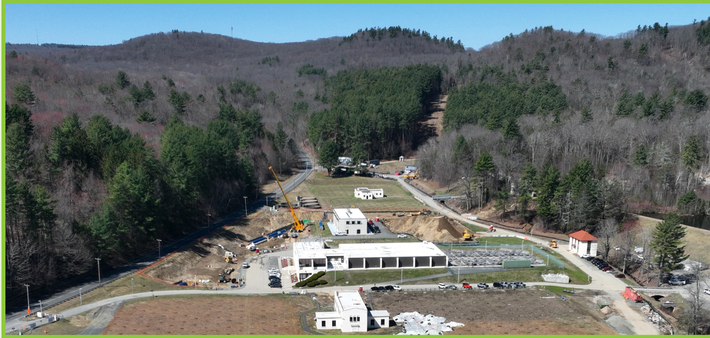
Construction of the new West Parish Water Treatment Plant underway at the site of the existing plant in Westfield, MA, April 2026.
